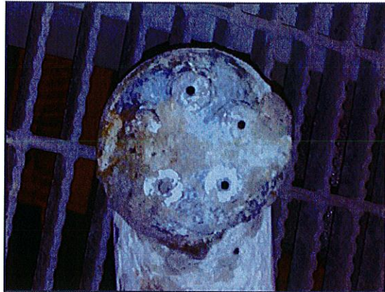
Photo 31 - Spray Nozzle - 3 of 5 Nozzles Plugged - PM Program Lacking
