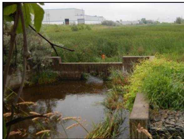
Upstream view of the outlet structure of an on-line quantity-control stormwater management pond
