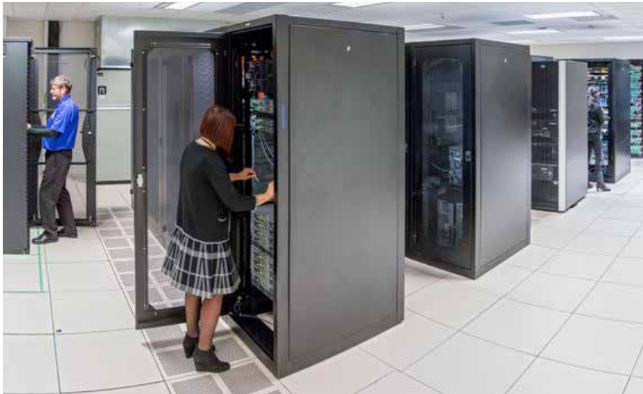
Figure 14: Regional server rooms. Cloud computing allows for data and applications to be centrally located and accessed by multiple devices.
